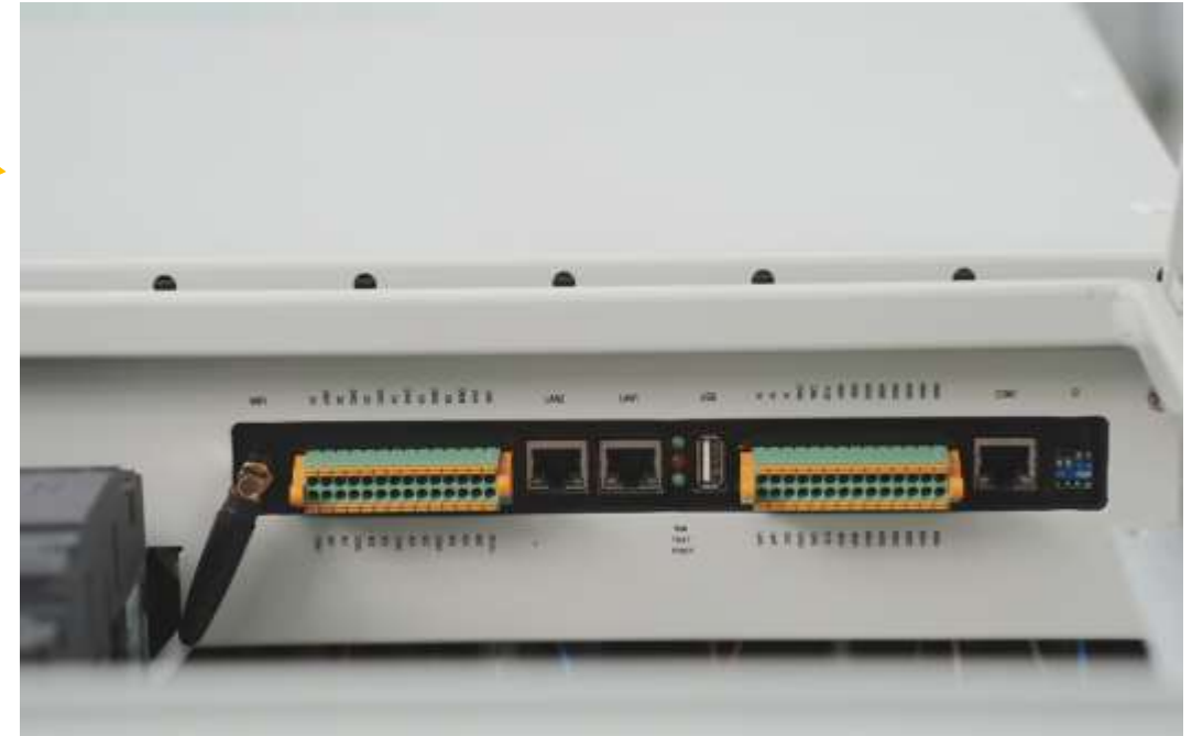
ATS communication port
